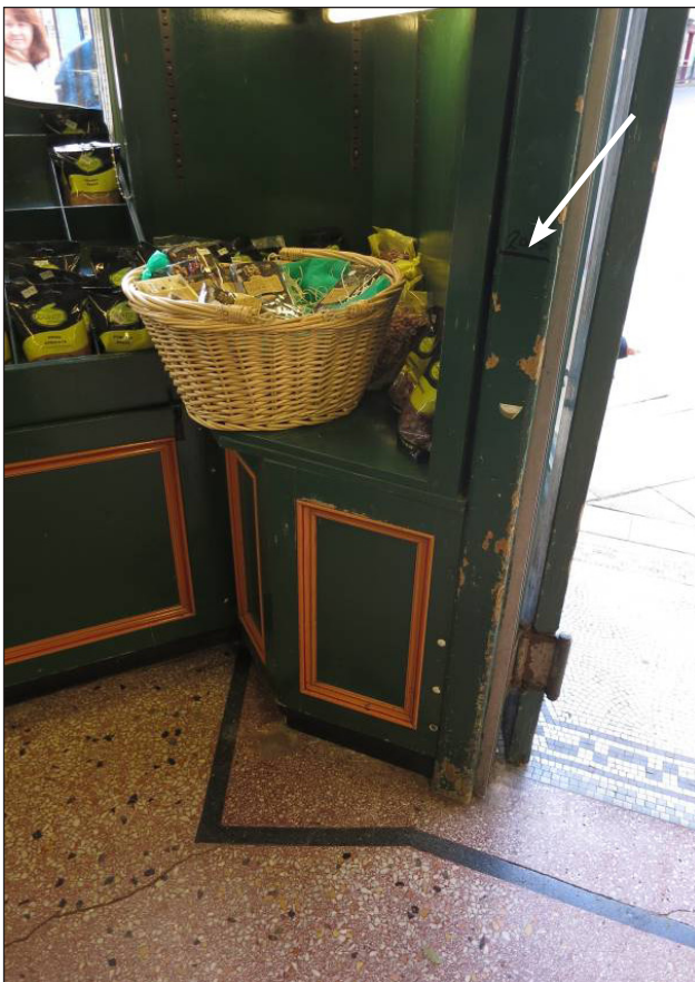
Figure 3: Arrow indicates the approximate depth of water above ground floor level.
