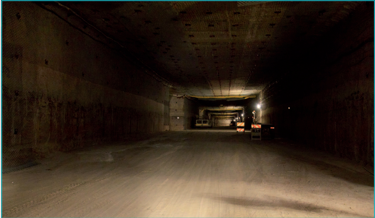
Figure 3.7: Underground facilities at the WIPP plant in New Mexico (source: WIPP)
