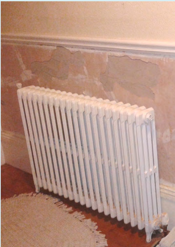
Some areas of skirtings, such as behind radiators, were not removed.
