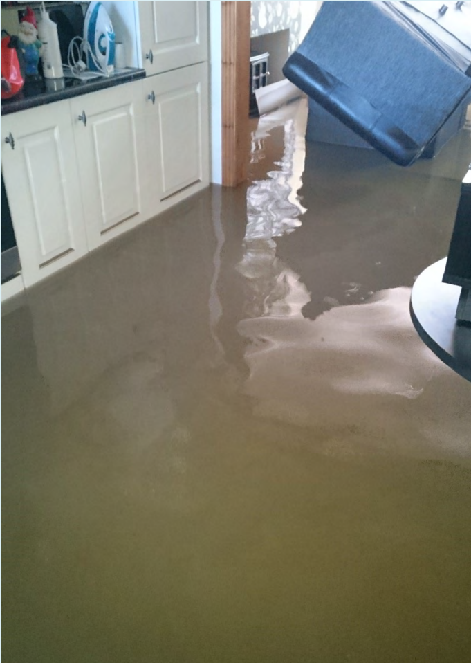
Flooding badly affected the kitchen and bathroom. The householder tried to move items like sofas above the flood water.
