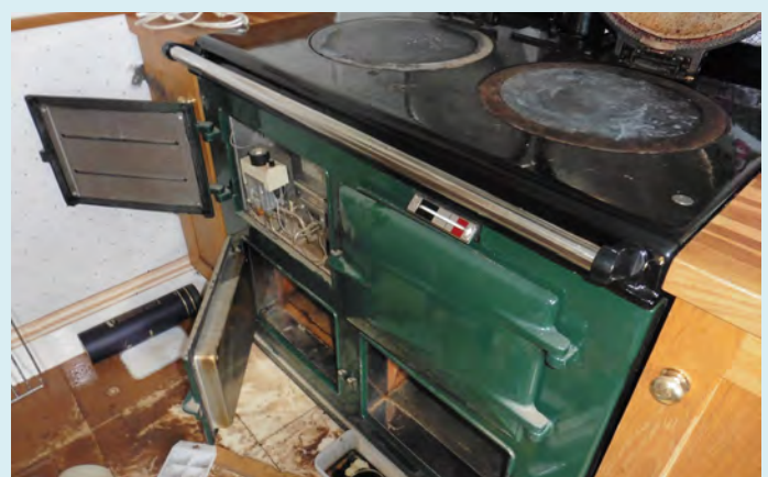
The AGA had to be replaced again after showing signs of rust.
