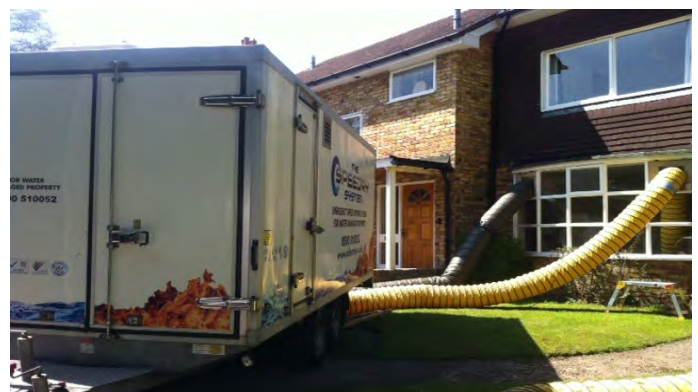
Above: speed drying trailer
